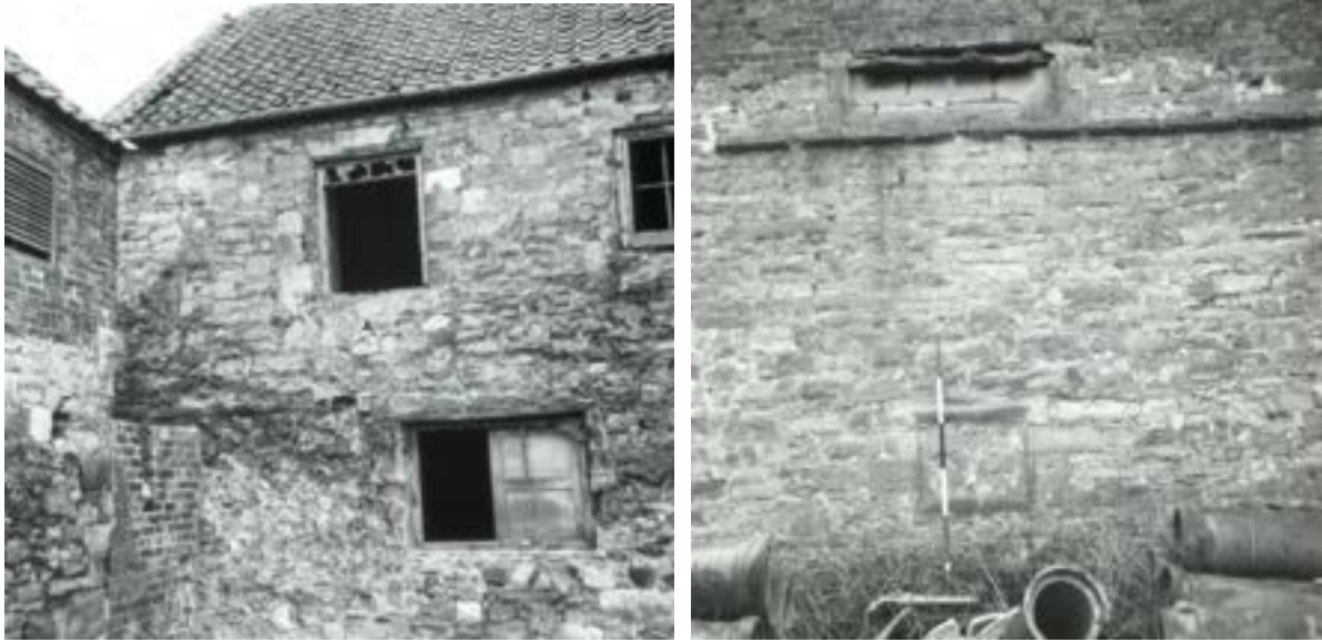
Figure 35: (a) The south side of the farmhouse, at the west end. Note the blocked first floor doorway, and the faceless stonework below. (b) The central section of the north wall, showing the small ground floor window, the string course, and the base of the two-light dormer window.
