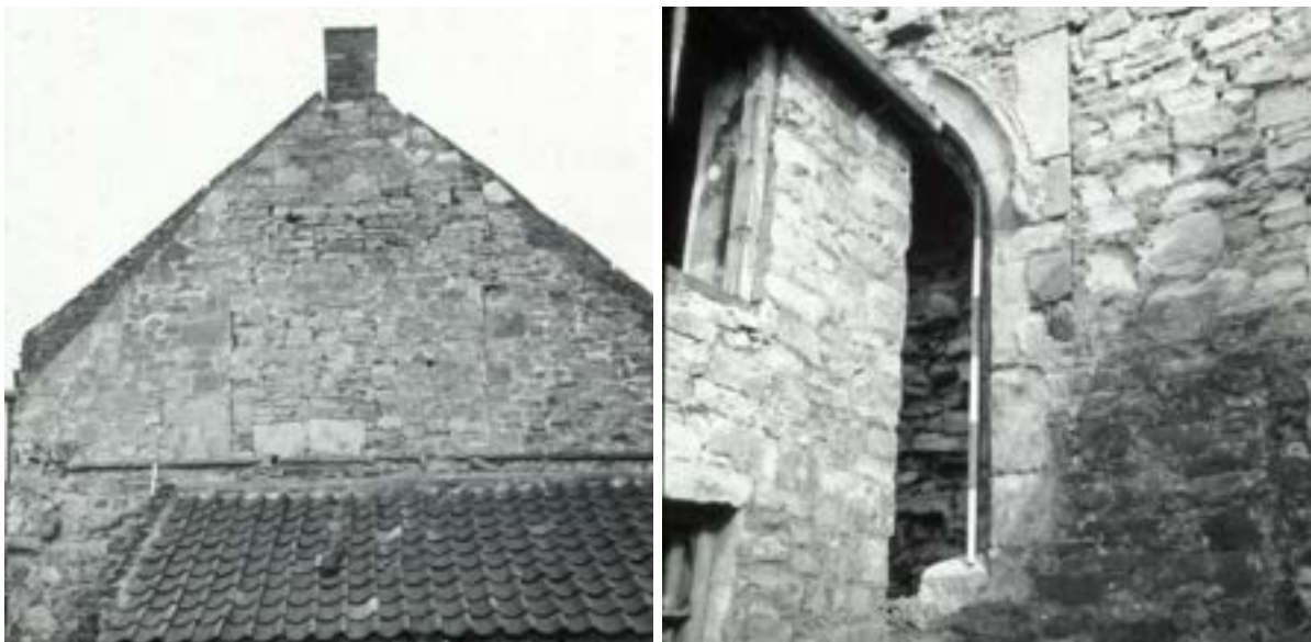
Figure. 34: (a) East gable showing raised and trimmed gable and blocked east window. (b) Blocked doorway in west gable before demolition of adjacent farm building. Also showing dressed quoins to the right of the doorway arch.
