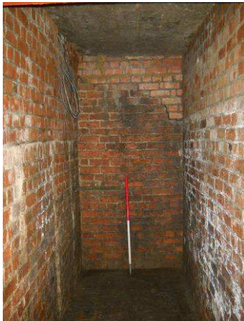
Figure 25: Air Raid Shelter Manor Croft, Hart, west side of shelter, note scar of previous barrel vault on end wall
