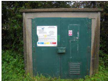
Fig 33: Burns Close, Water Pressure Booster Station, Structure B/X1
